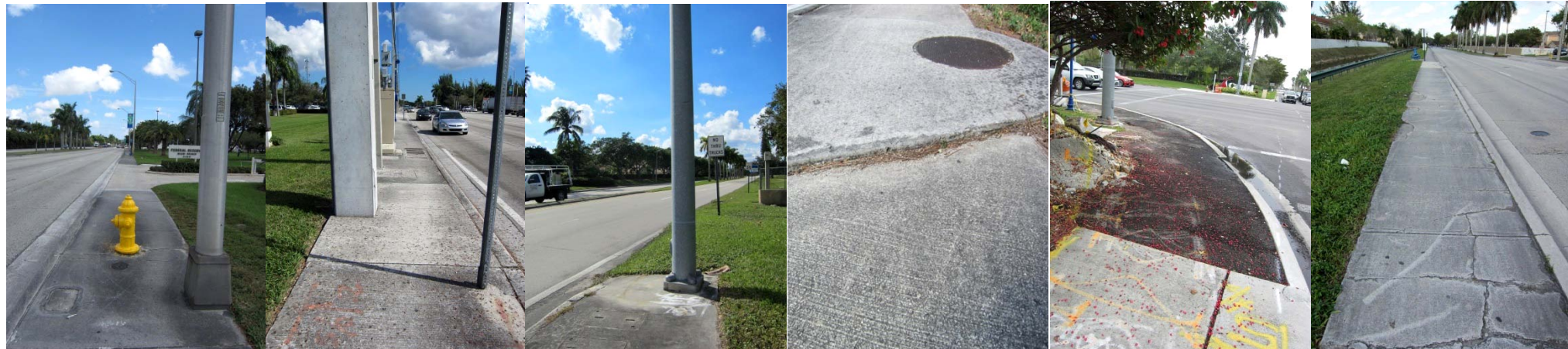
Issues encountered during a Field Analysis included (From Left to Right): Non-ADA compliant sidewalks, infrastructure obstacle course, missing sidewalks, uneven sidewalks, post maintenance issues, cracked sidewalks
